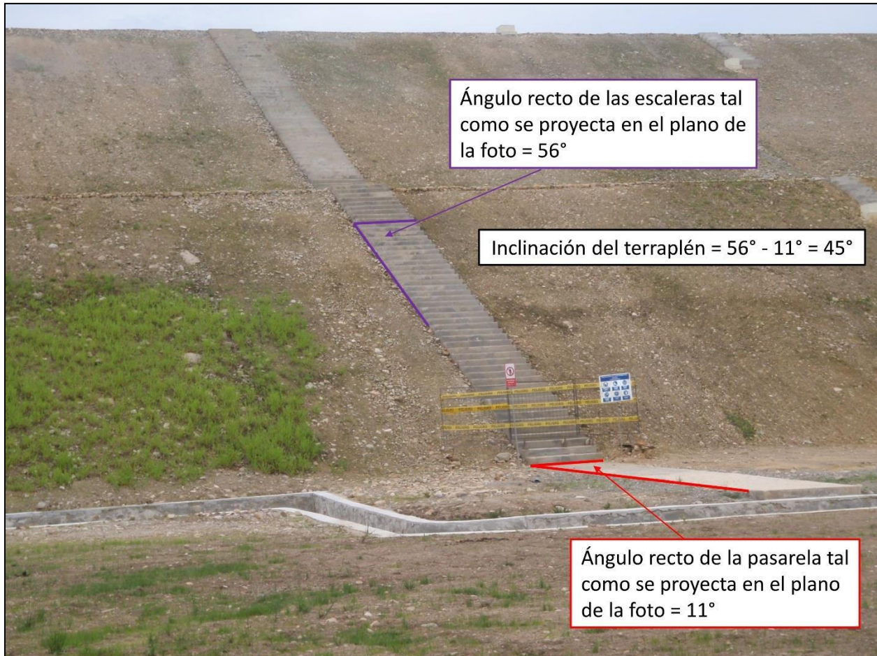
Figure 17. The initial embankment for the Quimi tailings dam has a slope of 1V:1H (45°). This is inconsistent with the design assessed by Knight-Pièsold (2007; see Figure 10) and both Environmental Impact Studies, which stated that the slope would be 1V:2H (26.6°). A slope of 1V:1H is considered the maximum critical angle to prevent internal erosion of the dam without any margin of error (factor of safety = 1,0). In contrast, according to the US Army Corps of Engineers (USACE, 2000), "for sand levees, a downstream slope of 1V at 5H [11.3°] is considered sufficiently flat to prevent seepage damage exiting the downstream slope [internal erosion]". Photo taken by the author on 6 November 2018.
