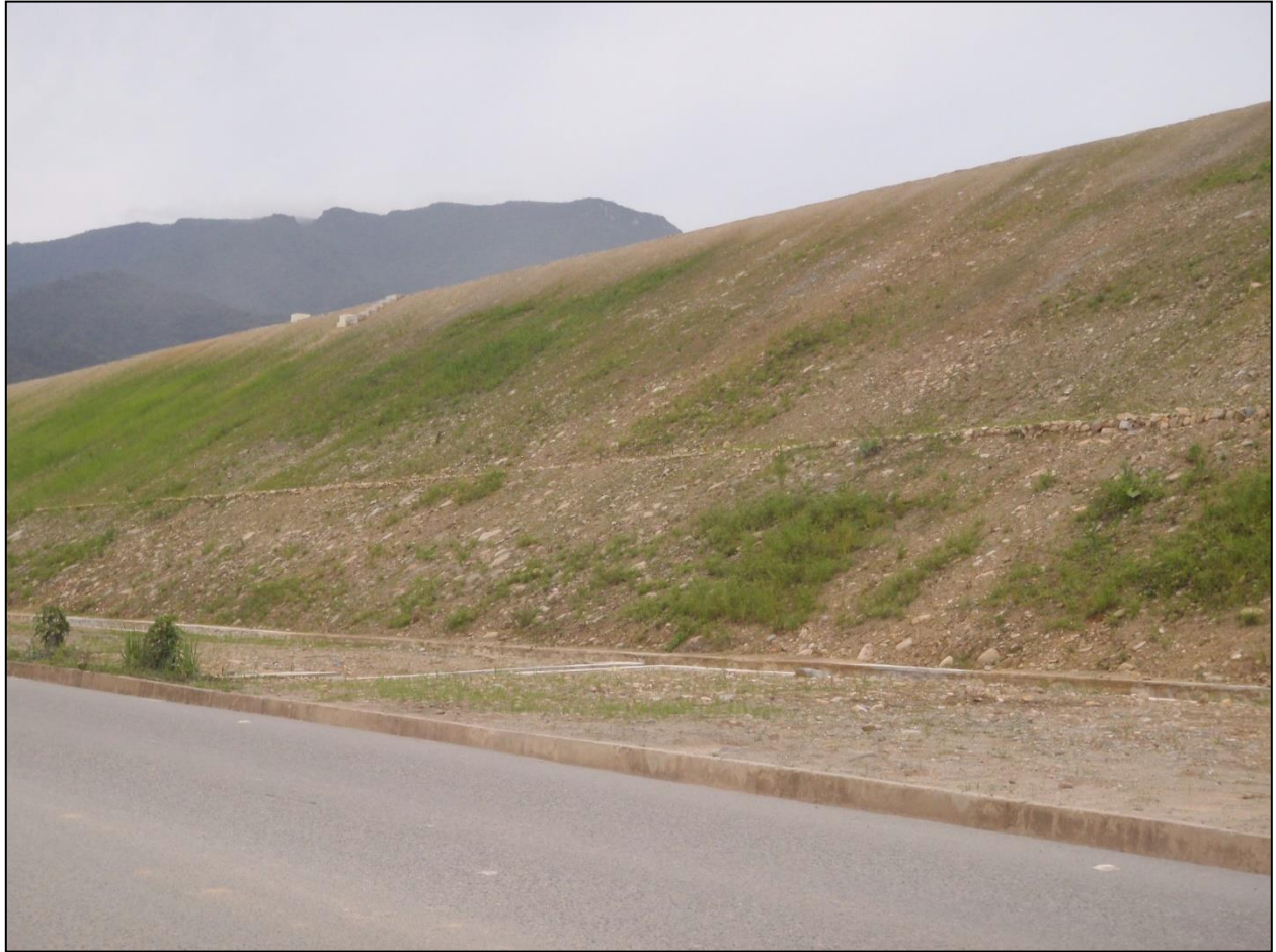
Figure 16. The initial dam for the Quimi tailings dam was built at the edge of the road, the other side of which is the river Quimi (see Fig. 11). Since it is not possible to advance the dam further in the downstream direction, the intention must be to construct the entire dam using the upstream method (compare Figures 5a-c). This is inconsistent with the design assessed by Knight-Pièsold (2007) and both Environmental Impact Studies (Walsh Scientists and Engineers, 2010b; Cardno, 2014a), both of which included centreline construction for the Quimi tailings dam. Tailings dams constructed by the upstream method are more susceptible to failure by both earthquakes and flooding. Due to the inability to install impermeable layers (see Figures 5a-c, 8), their higher water content also makes them more susceptible to failure by internal erosion, static liquefaction and foundation failure. Photo taken by the author on 6 November 2018.
